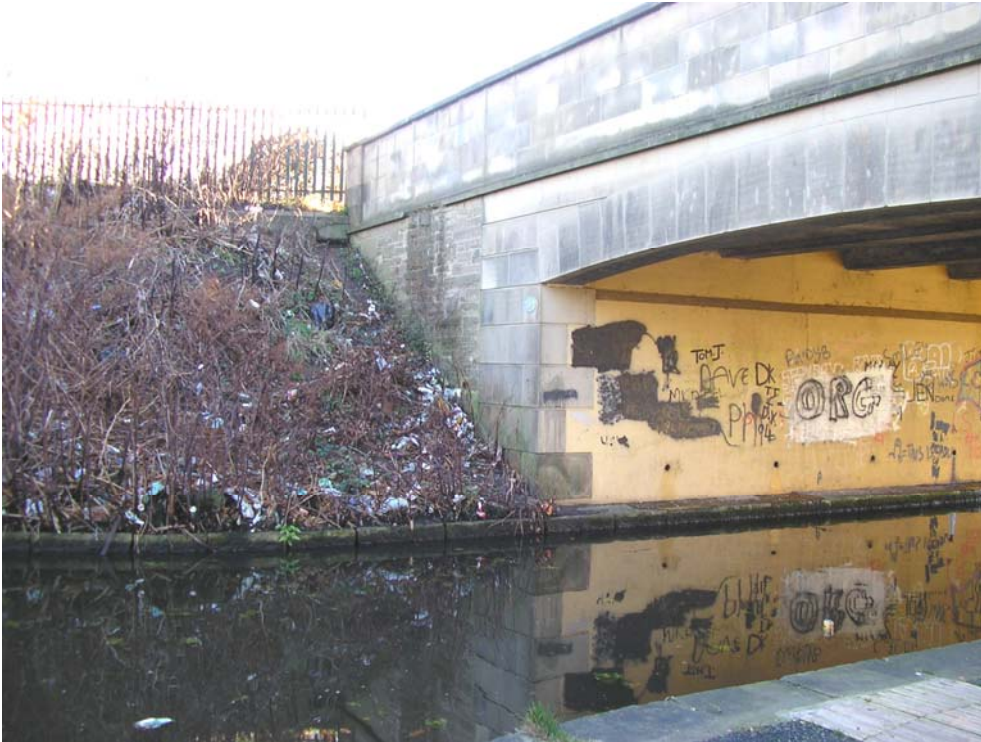
Photograph showing litter adjacent to bridge and graffiti.
